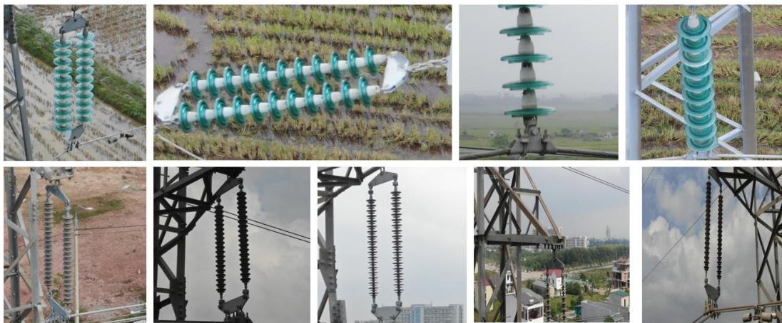
Figure 2. Example of insulators
