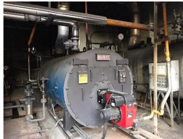
Figure 1. Boiler for producing hot water and steam
