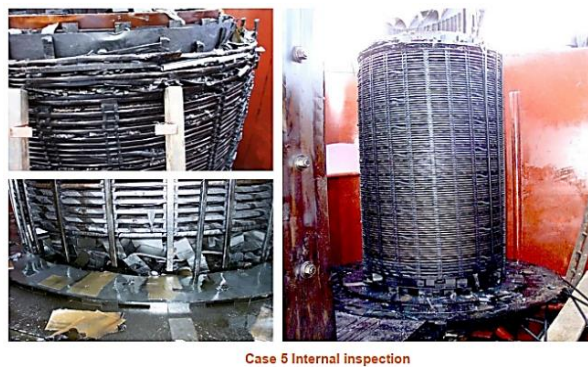
Figure 5. Twisting and loosening of the clamping fault.
