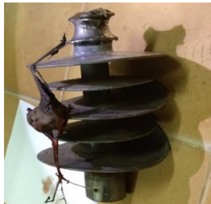
Figure 4. Bat causes S.C fault on isolated porcelain
