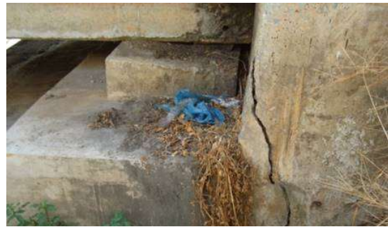
Figure 2. Large cracks appeared on head wall, wingwall of abutment
